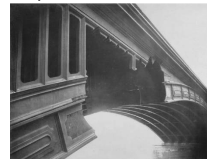
Photograph of Diamond damage; Rochester Bridge Trust.
